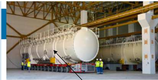
Air Liquide 4K Cold Box
